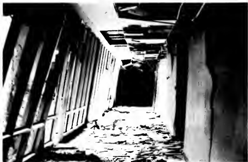
Photo 28. Fallen ceiling tile, first story of Medical Treatment Building. Glass was originally vertical.
